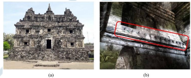
Fig.7. (a) Exterior of Sari Temple and (b) the holes for the wooden floor beams in its interior (author's document).
