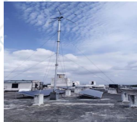
Fig. 1. Solar-wind hybrid microgrid of 7.5KW Capacity.
